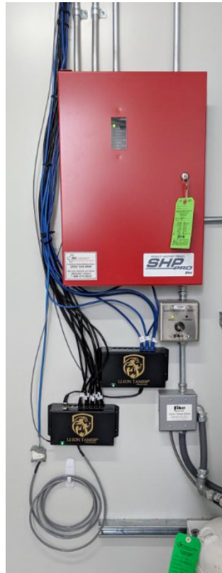
Figure 6: solar power plant BESS
