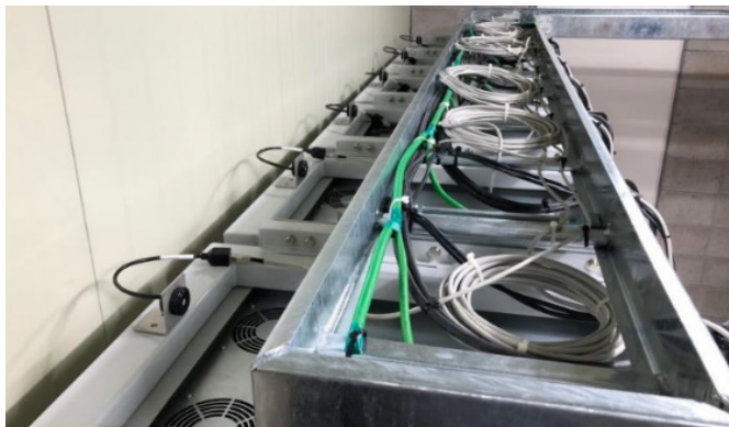
Figure 7: commercial facility battery room
