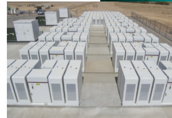
Figure 1: Multi-cabinet utility-grade BESS
