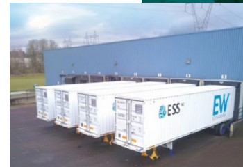
Figure 2: Containerized behind-the- meter BESS
