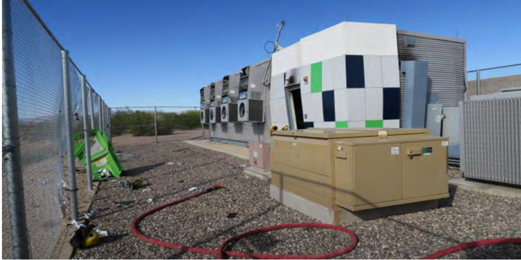
Figure 4.18: Photograph of firefighter helmets and the door to ESS removed during the deflagration [6].
