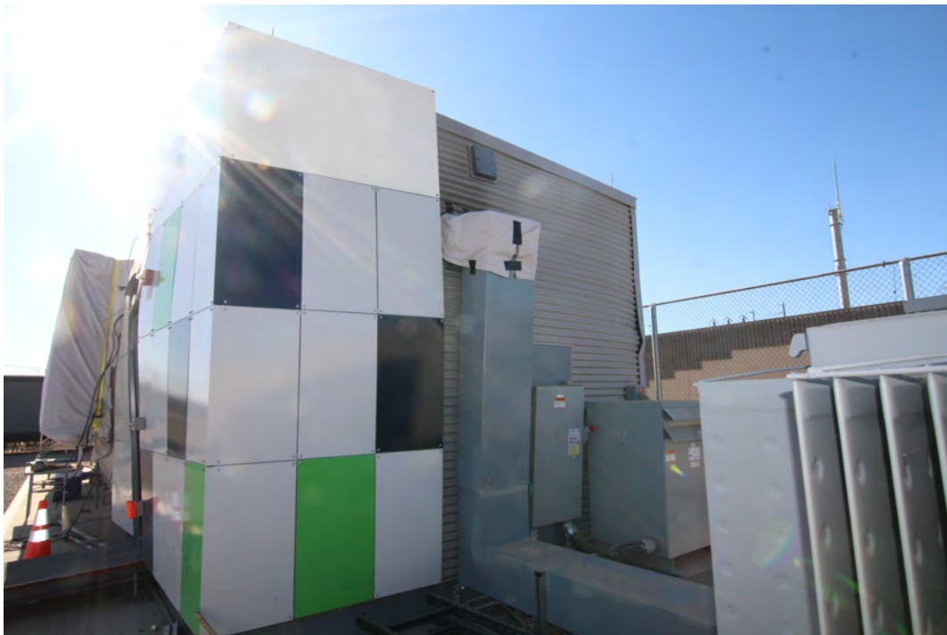
Figure 4.4: Photograph of the ESS after the incident from the northeast [13].
