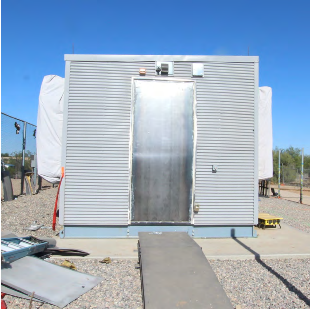
Figure 4.6: Photograph of the ESS after the incident from the southwest [13].
