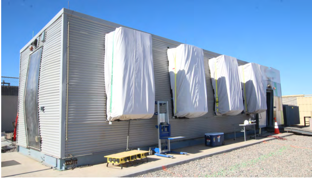
Figure 4.3: Photograph of the ESS after the incident from the southeast [13].
